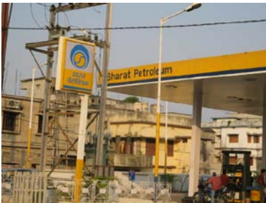
Fig 12.1: Electric Transformer and Post near Petrol Pump
