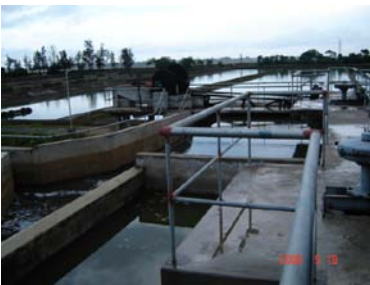
Fig 8.8: A view of the sewage treatment plant of 33 MLD capacity located at Matgajapur.
